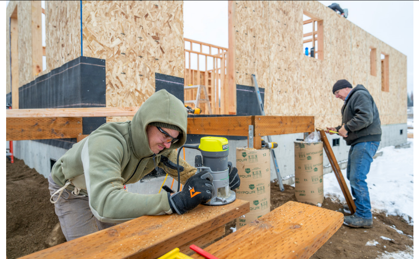
MDS Crew Leader Nathan Fisher and volunteer Michael Eigsti construct the deck of a house.
